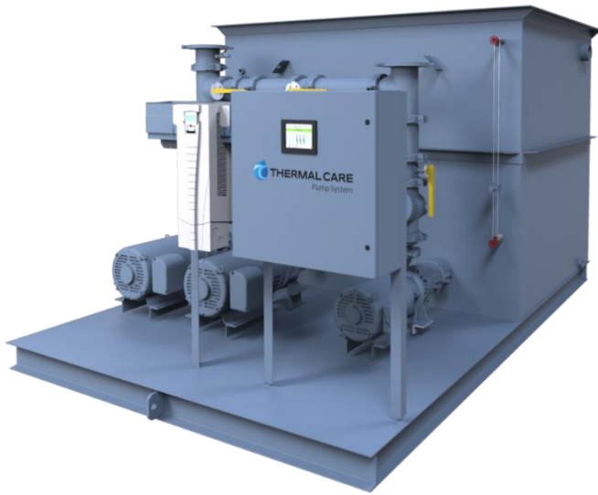
Typical system with 3-pumps, process pump VFD, and control panel with PLC and color touch-screen
